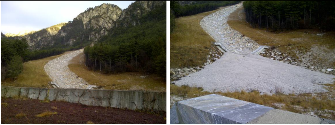
Figure 2 and 3 Conformation works for slope stabilization along debris flow channel in the Malborghetto village, December 2011.
