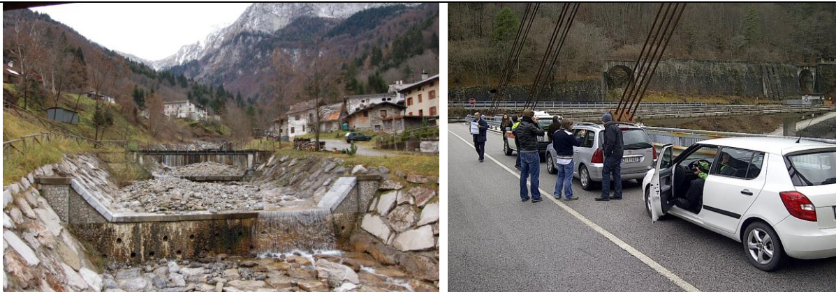
Figure 26. (Left) Protection works carried out over the affluent of the Fella river where we can observe the online structures for retention of sediments and slope protection along the stream channel. December 2011.
