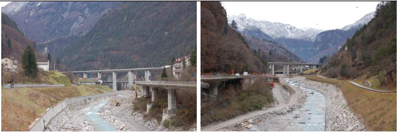
Figure 24 and 25. Overview from the bridge perspective of the reconstruction and protection activities after the 2003 event. December 2011.
