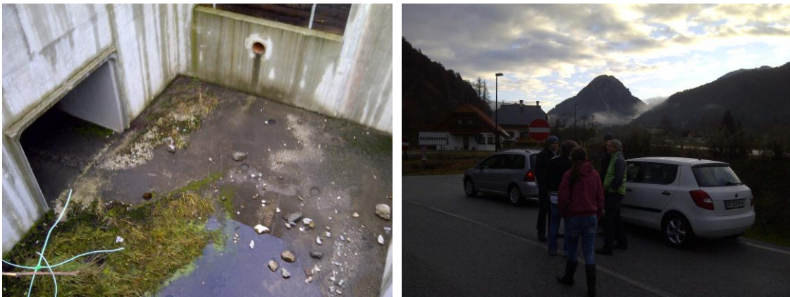
Figure 4 and 5 Hydraulic structure that conducts the flow from the conformed slope channel to the Fella river below the road, December 2011.
