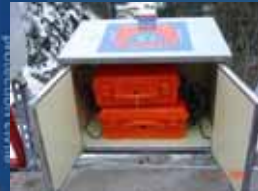
Steel-boxes to avoid air moisture
